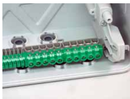
Earth terminal block: screw terminals (depending on the type of cabinet)
